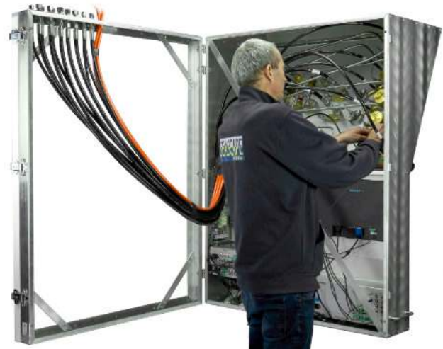
easy access for maintenance
